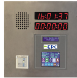
OPERATING ROOM CONTROL PANEL
