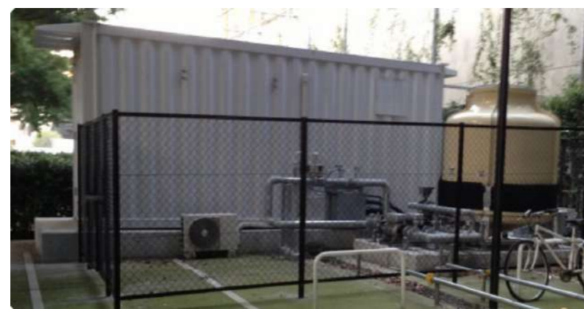
Fig. 3. Exterior view of TSUBAME-KFC: evaporative cooling tower right next to the 20-foot container for complete lights-out operation and low waterpump power
