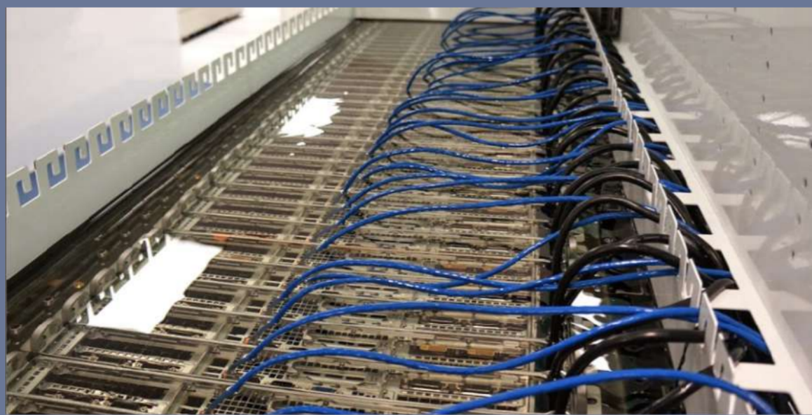
GRC's ICEraQ cooling system in action
