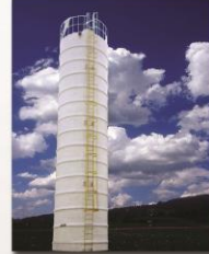
Vertical HCL Storage Tank
